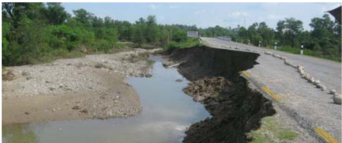
Damaged road in the Far West of Nepal
